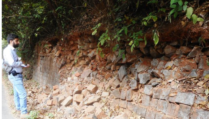
Photo 14: Disruption of retention wall along SK border -Kalasa road section. TS O/3
