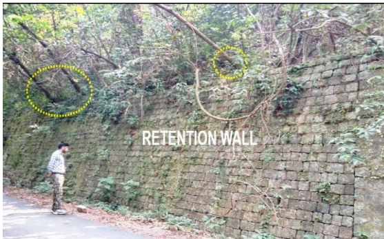
Photo 15: Bulging of retention wall with inclined vegetation growth along SK border -Kalasa road section. TS O/3
