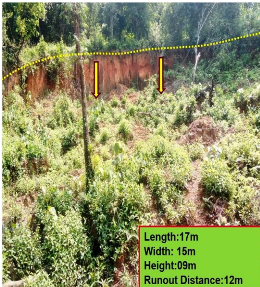
Photo 18: Subsidence along Bhagavati - Kalasa Road section (NH13). TS O/3
