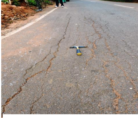
Photo 13: Road cracks adjacent to a failure along NH-13 towards Nemmaru. TS O/3
