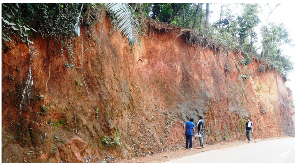
Photo 3: Extensive cut slope Near Bhagvati Nature camp. TS O/3
