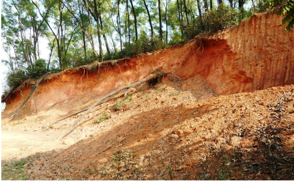
Photo 4: Extensive cut slope near Makkimane Extensive cut with overturned trees. TS O/4
